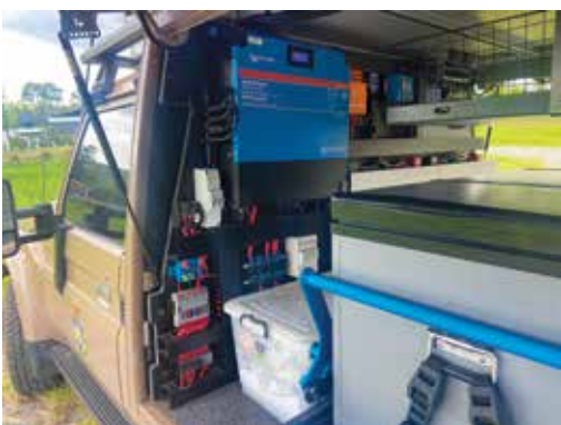
Inverter & other equipment
